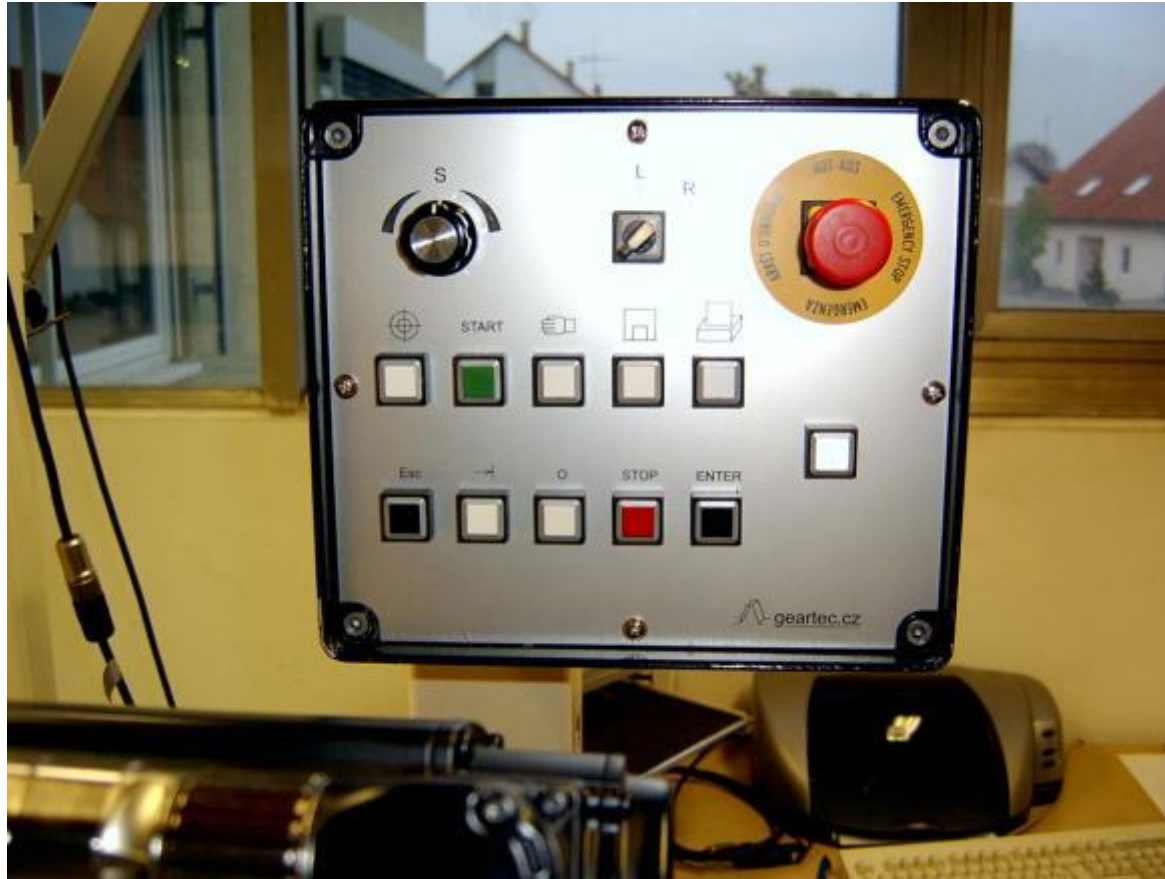
New control panel
